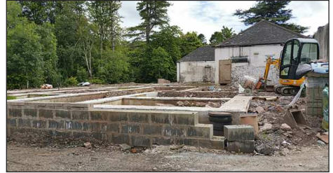
Above – the extension to the original Grey Lady. Very deep foundations were extremely costly.
